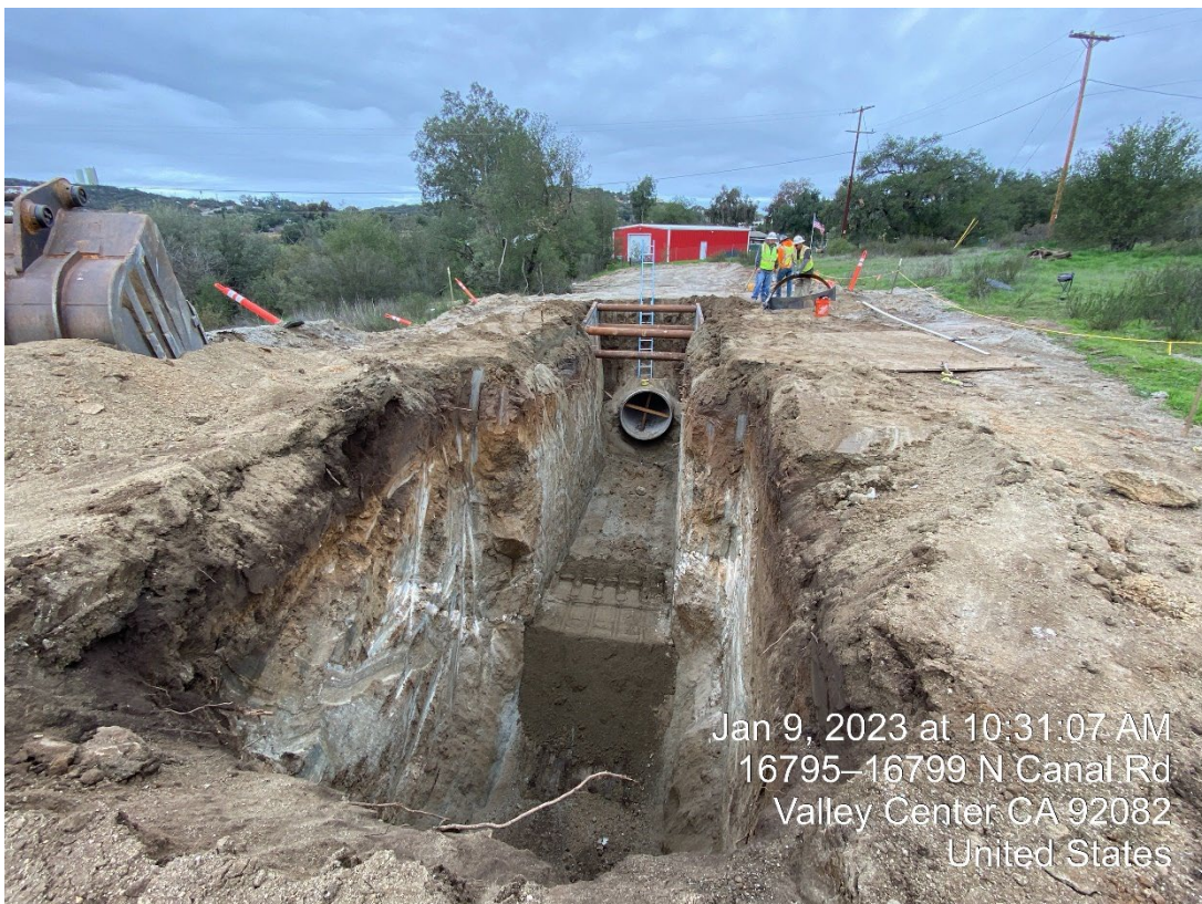
Excavating trench to the north of the tunnel to continue with pipe installation from station 84+30
