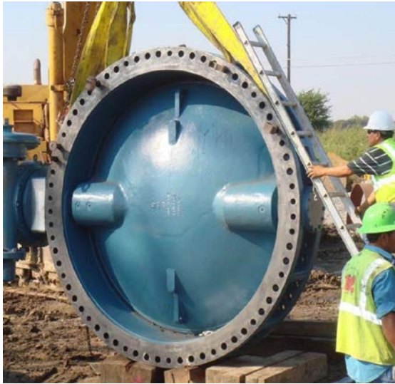
SDCWA Isolation Valve Project
