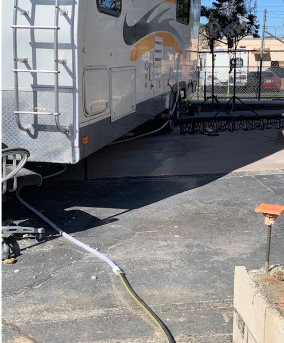
Illegal hose connection connected to trailer hose at 170 Eucalyptus February 6, 2019
