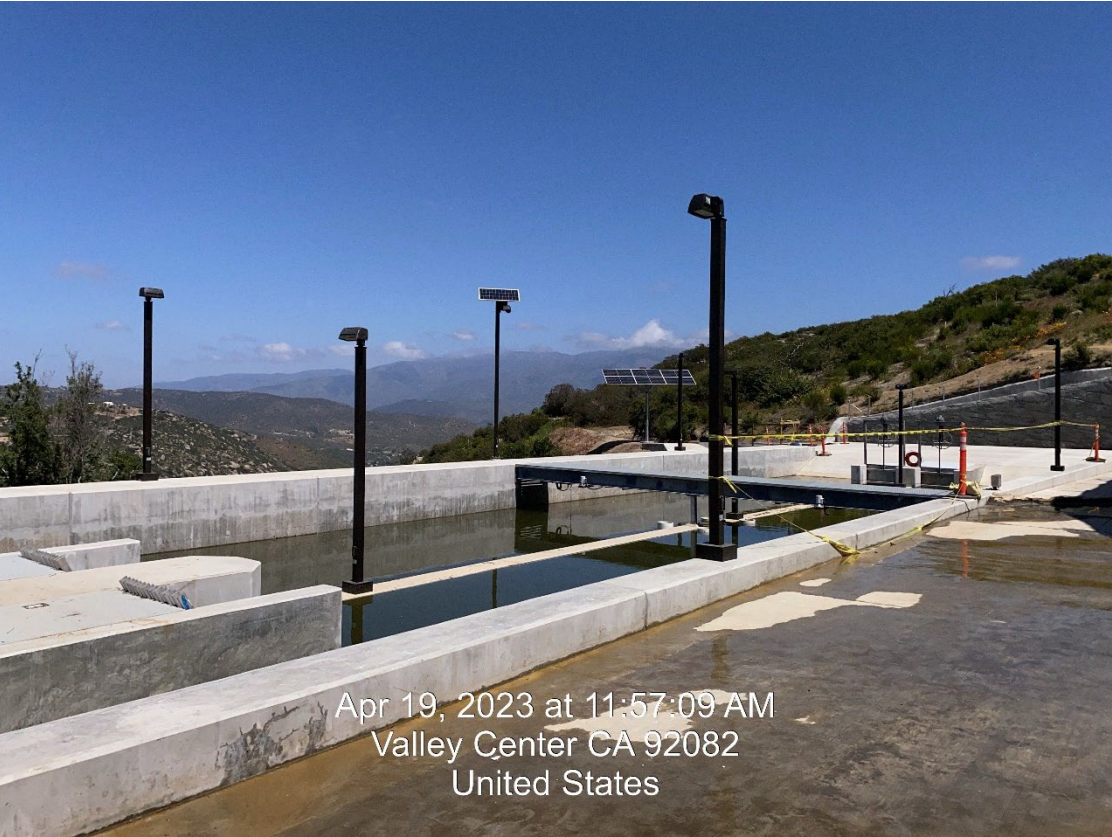
Desilting basin with all light, camera and solar device
