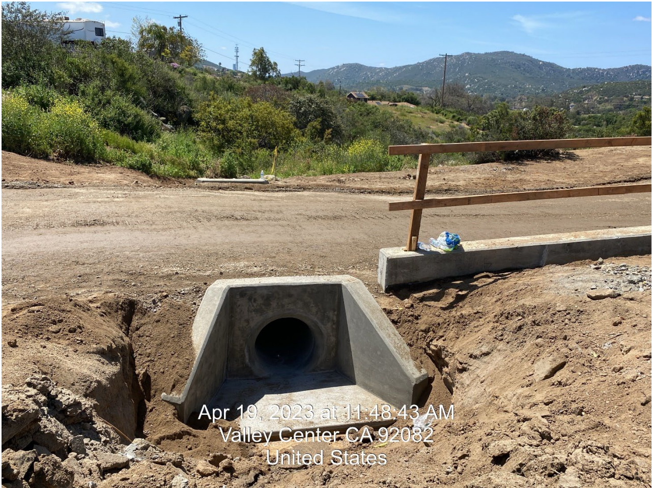
24" RCP pipe and headwalls
